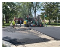
Crews pave over the final stretch of the Country Club Highlands project.
