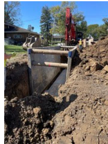
Installation of storm sewer being completed along Roosevelt Road in unincorporated Lombard.
