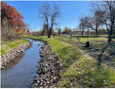
A freshly restored portion of Winfield Creek, featuring a stabilizing rock toe along the bank and new trees planted in the adjacent wetland area.
