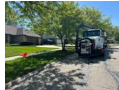
SWM equipment and personnel deployed to Peters Court in Downers Grove Township to assist with flushing out a blocked sewer.
