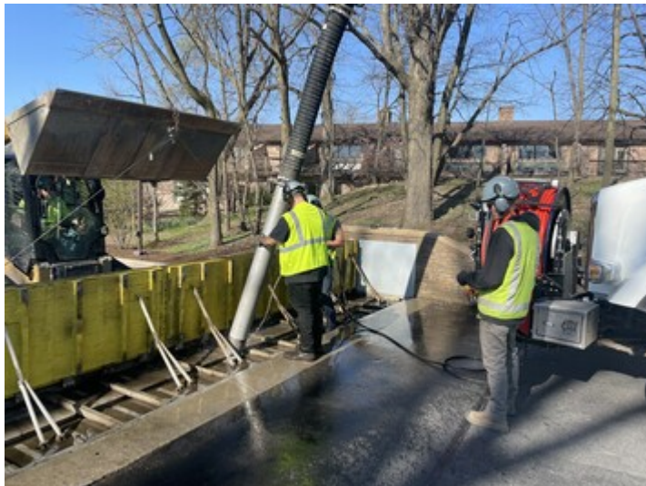
SWM Maintenance Crew members clean a flood gate in Hinsdale to ensure operation during an emergency event.
