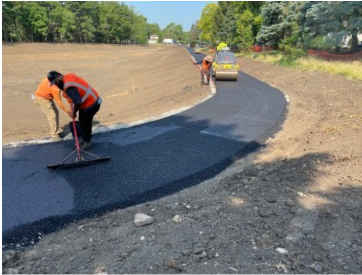
V3 Construction crew install an asphalt pedestrian path around the Main Street Flood Storage Facility.
