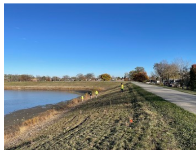
SWM staff walks the Armstrong Park Reservoir to inspect the dam. Flags are used to mark animal burrows and woody plants that could compromise the function of this dam that protects a portion of Carol Stream.
