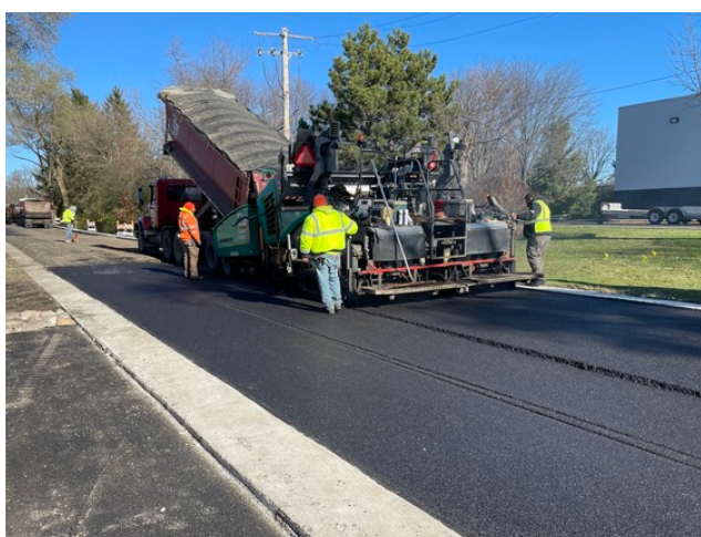
Work crews lay down fresh asphalt over the new storm sewer system installed in unincorporated Lombard as part of the Luther High Ridge Flood Relief project.
