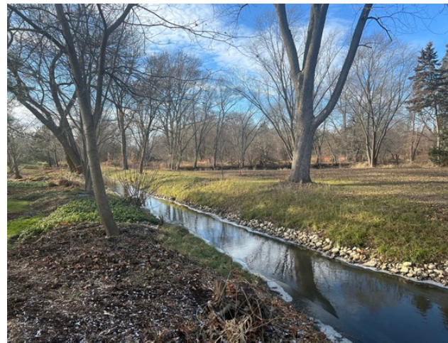
A portion of Winfield Creek has a new lease on life after SWM completed its streambank stabilization project, funded mostly through a grant from the Illinois Department of Commerce and Economic Opportunity.
