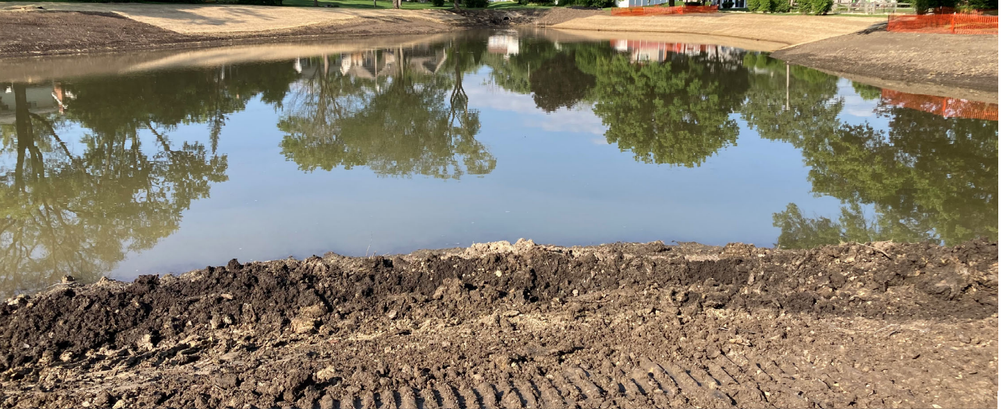
Lufkin Pond Drainage Project in Villa Park mid-progress, funded entirely through ARPA.
