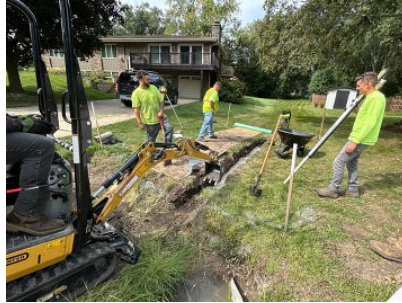
From the Annual Report: SWM field crews work to repair a section of the Cotuit Court drainage system in unincorporated Glen Ellyn, one of many Shared Services projects completed by the Department in 2025.
