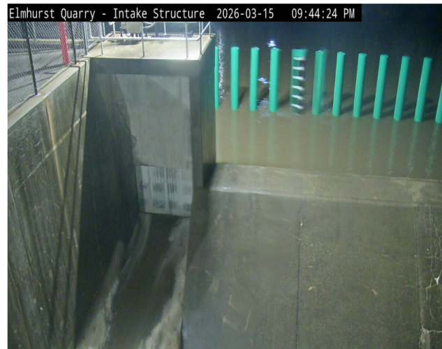
A camera feed from the Elmhurst Quarry Intake Structure shows water flowing in at 9:44 PM on Sunday, March 15.
