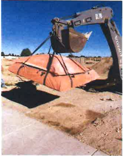
(C) TEMPORARY CONCRETE WASHOUT
